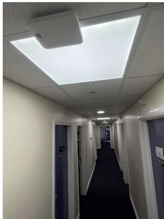
Photograph Six – LED Light Fittings
