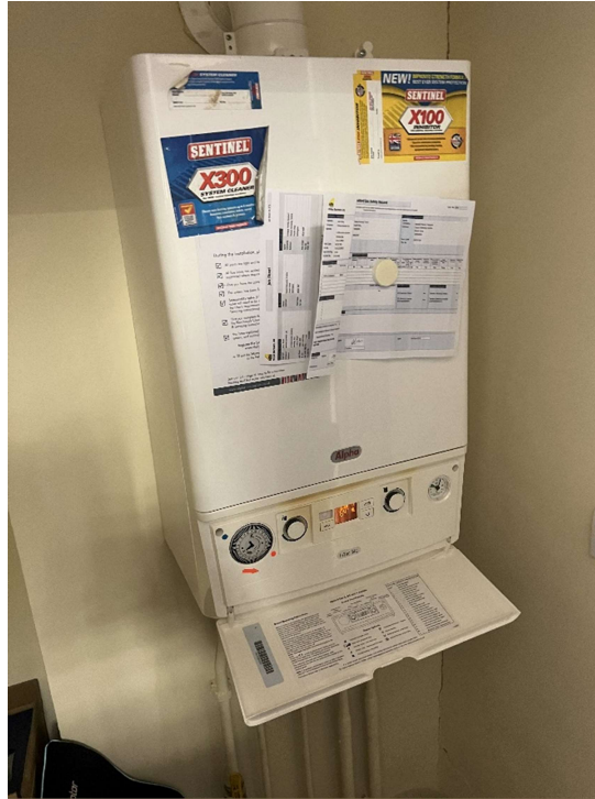
Photograph One – Gas Fired Condensing Combination Boiler
