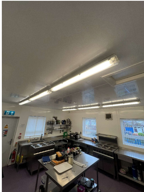
Photograph Five – Fluorescent Light Fittings
